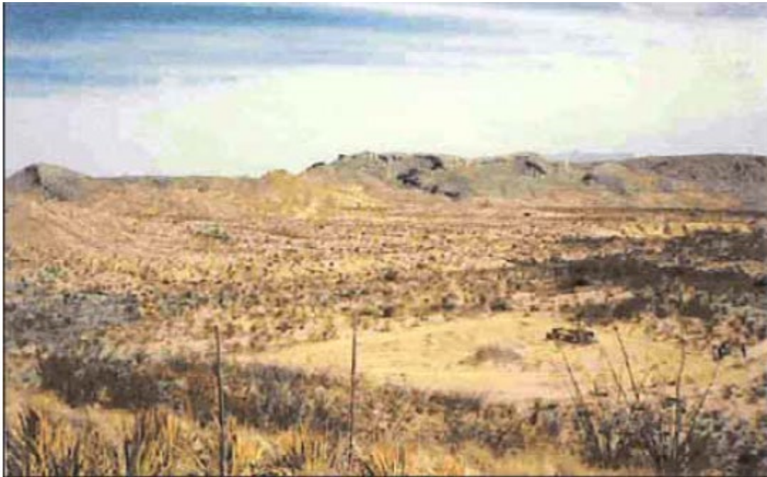
Our road grader operator doing some land clearing at the cooks' site
